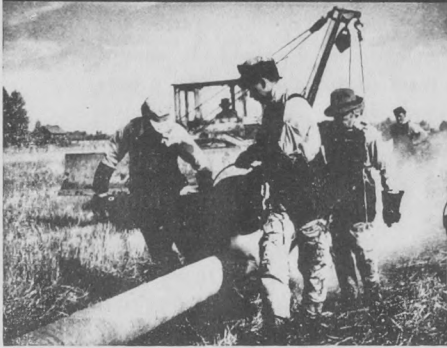
17 Before the pipe was laid in the trench and covered over a side-boom caterpillar tractor held it for an insulation crew which followed, tarring, wrapping, and tarring again
